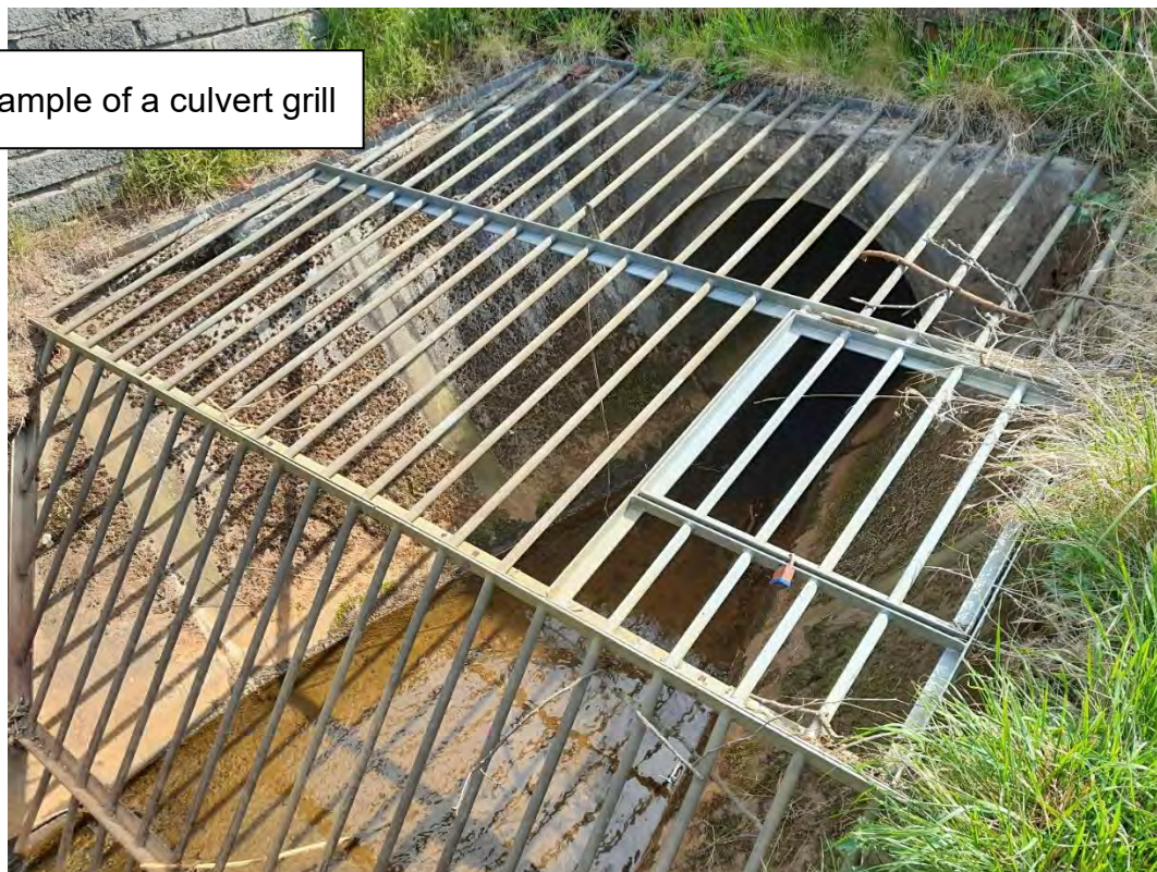
Example of a watercourse grill
