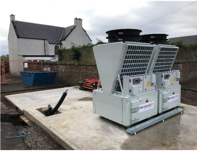
Heat pumps located on concrete base at Hill of Beath Primary School part way through construction. This site is now nearing completion.
