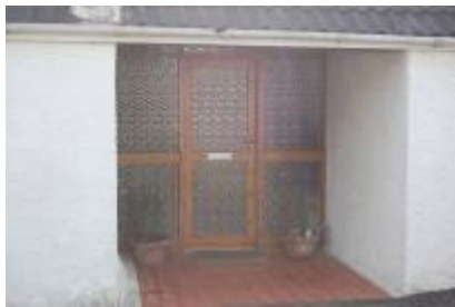
Inappropriate door replacement
