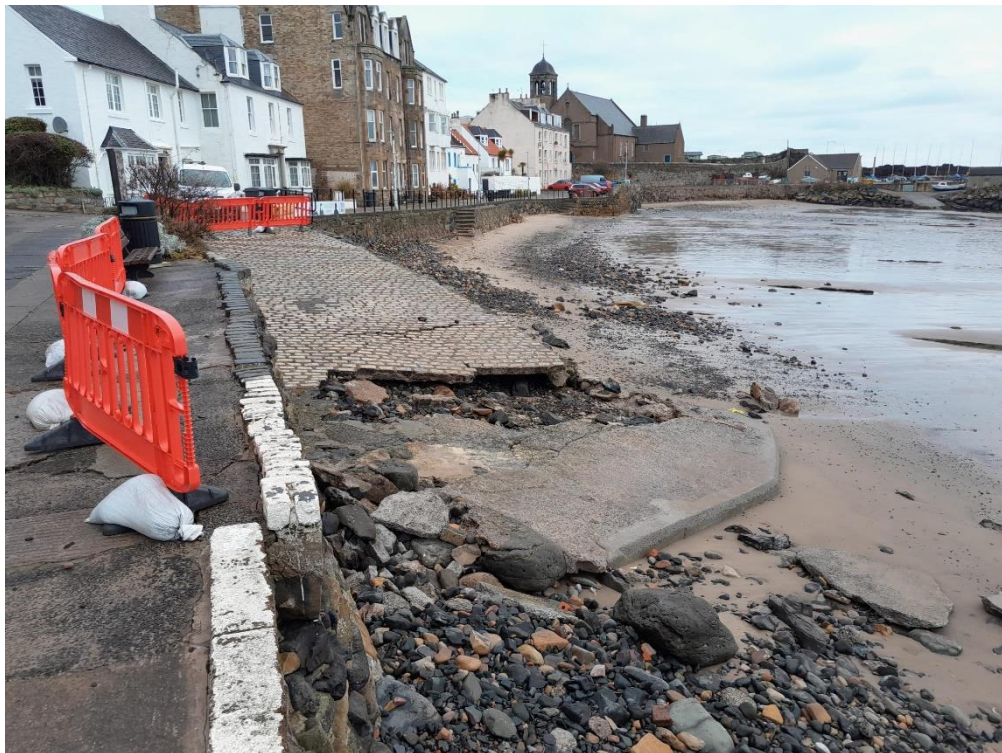
Figure 2: Slipway damage (17 November 2023)
