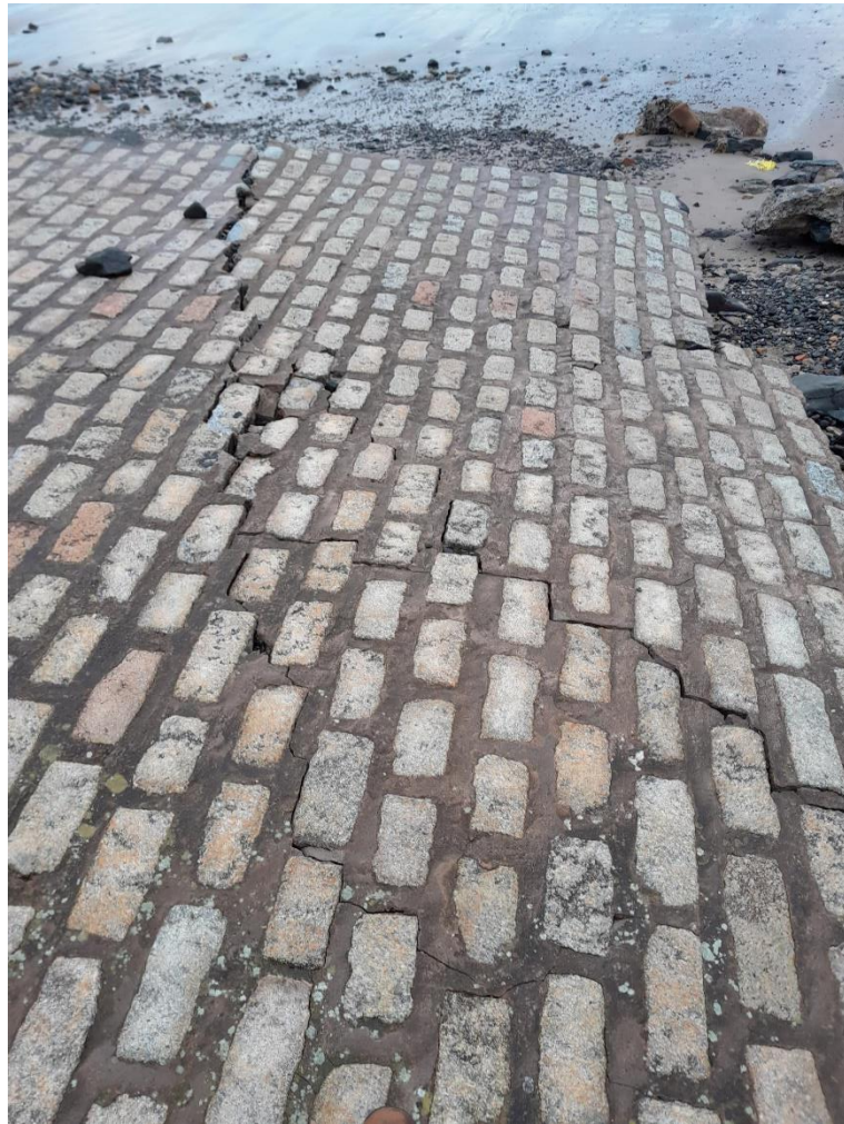
Figure 3: Cracks / Failure of Slipway (17 November 2023)
