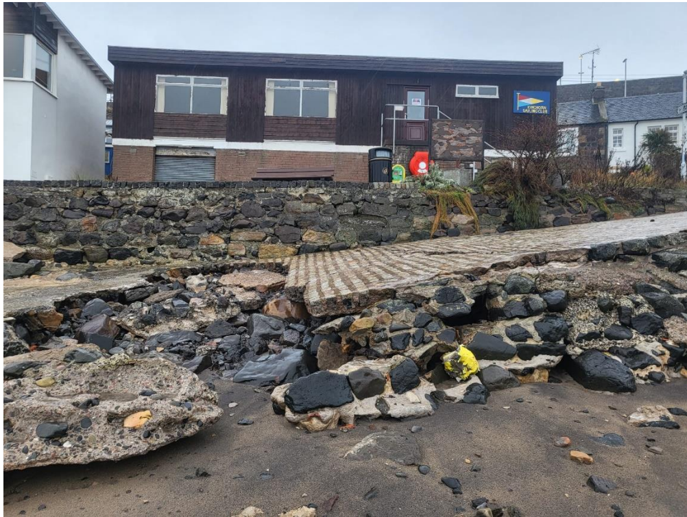
Figure 1: Slipway damage (01 November 2023)
