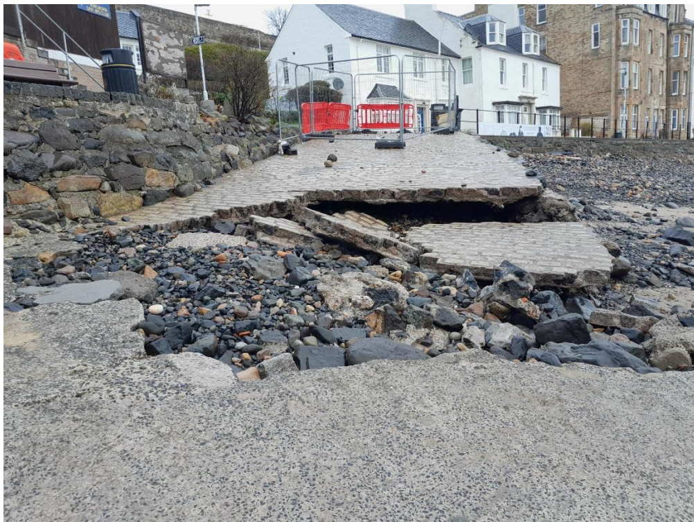
Figure 4: Slipway Damage (14 March 2024)
