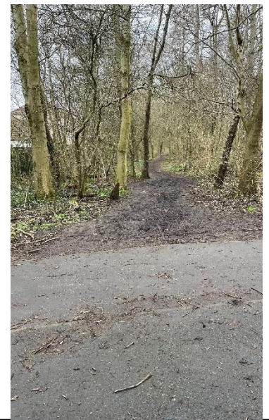
Condition of footpath – some woodland debris
