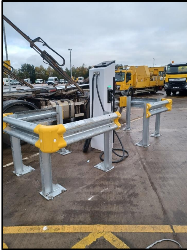
Figure 3 - 150kW charger recently installed and commissioned at Bankhead Depot, Glenrothes
