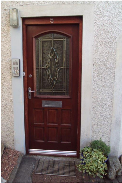
Modern replacement door of inappropriate design and finish.
