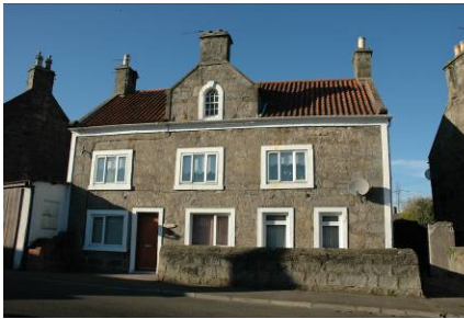
Non-traditional windows adversely affecting character of B Listed property, Keith Street
