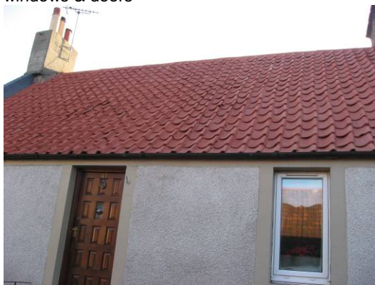
41 Keith Street: gaps between pantiles filled and overpainted, chimney cope lost, dry dash walls, non-traditional replacement window and door
