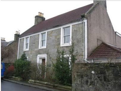
60 Kilbagie Street, B listed, clay pantiles replaced with concrete tiles of incorrect profile and colour
