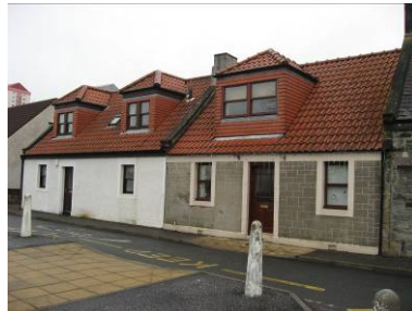
24-26 Kirk Street, C(S) Listed: whilst these dormers may seem preferable to the illustration of those in Kilbagie Street, their detailing is very heavy and they dominate the roof; more care is required
