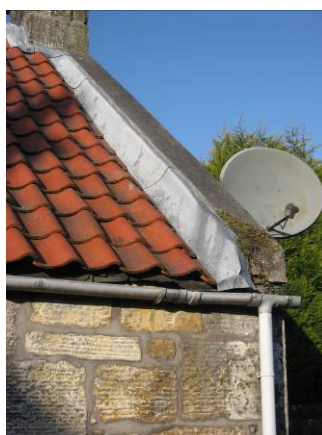
8 Bank Street: original pantile roof but concrete over stone skew, plant growth on skew, Upvc rainwater goods, cement pointing, satellite dish
