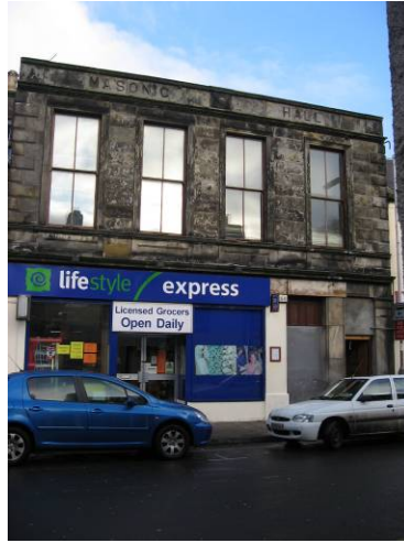
10 Elphinstone Street, C(S) listed: unsympathetic sign and shop front, poor treatment of doors and door ways, unnecessary painting of ashlar stone
