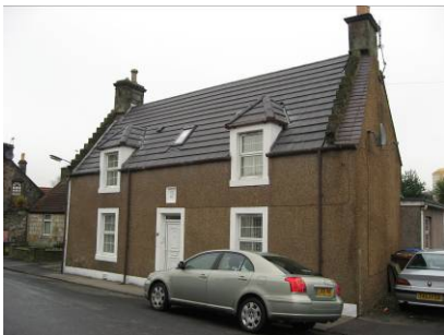
24 Kilbagie Street, B listed, natural slate replaced with concrete tiles in December 2008
