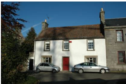
Upper floor traditional timber sash and case windows, ground floor window openings widened in 1920s for new metal casement window, 23 Forth Street. See also section 3.4.2.
