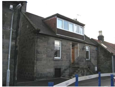
52 Mercer Street, C(S) listed: concrete roof tiles, unsympathetic dormer extension, Upvc replacement windows, concrete steps and inappropriate handrail
