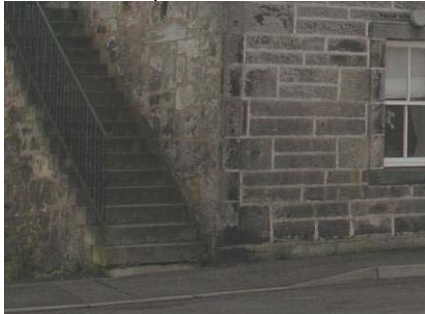
1,2 Forth Street, loss of stone step in tarmac when pavement installed
