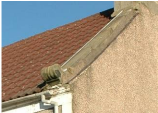
Plain skew with scroll skew putt with ropework detail on 60 Kilbagie Street
