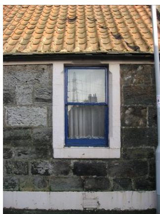
8 John Street Street: in need of repair but original timber sash & case window, pantile roof & cast iron guttering
