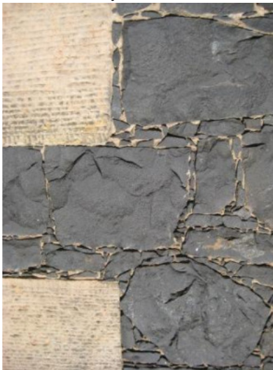
Dark whinstone rubble masonry contrasting with blonde droved sandstone outband by bats to window margins. Note the very narrow mortar courses with tight pinnings
