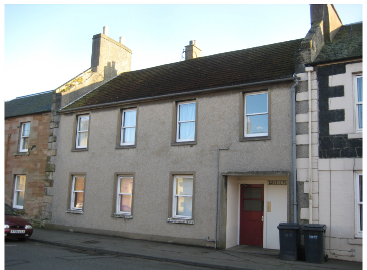
Dry-dash cement render; upvc windows; plastic rainwater goods; concrete roof tiles; varnished glazed recessed door
