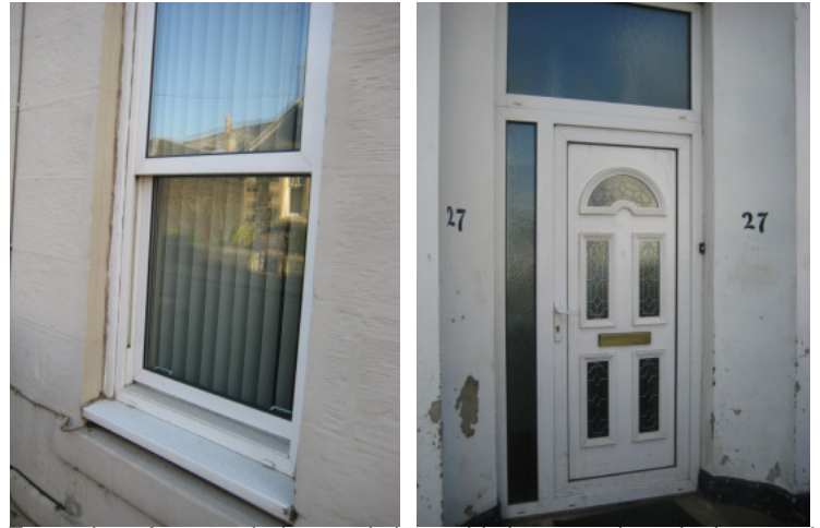
Examples of upvc window and door with inappropriate designs and detailing
