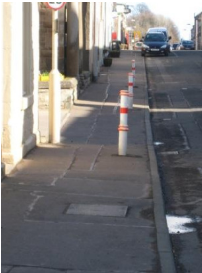
Typical patch repaired road and pavement surfacing. Note: unsympathetic design and painting of bollards; speed sign and litter bin
