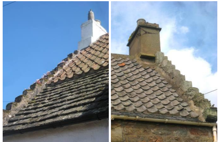
Typical East Neuk vernacular roof detailing: crow step gables; moulded skew-put; pantiles with slate easing courses. Note thackstone on right-hand chimney head.
