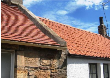
Historically and architecturally inappropriate plain Rosemary tiles (left)
