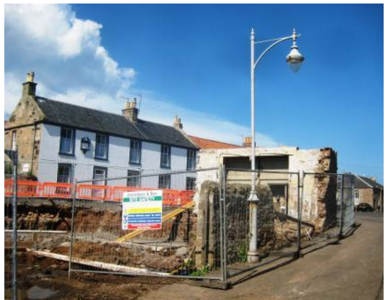
Listed mid-19 th century former lifeboat shed at Nethergate West. Unlawfully partially demolished.
