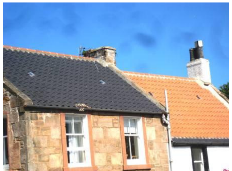
Examples of the different roof tiles and detailing above and left. Note traditional grey pantile left and modern imitation above.
