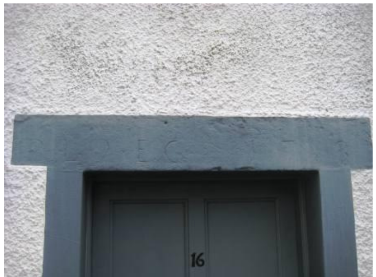
In example above, the modern film forming masonry paint may be trapping moisture and resulting in the accelerated decay of the
