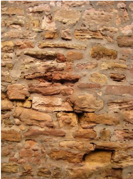
Accelerated decay of masonry due to effect of introducing modern cement mortars.
