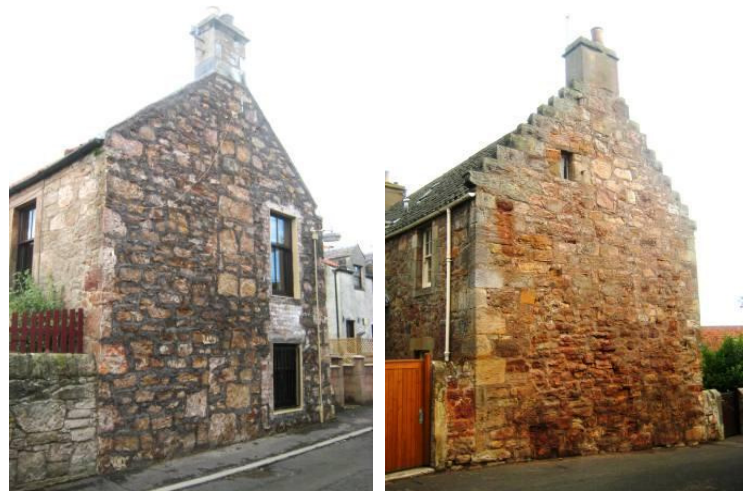
Left-Recently re-pointed gable wall using cement mortar. Right- similarly re-pointed gable showing signs of accelerated decay of stone and increasing concentration of moisture towards base (see detail above left).
