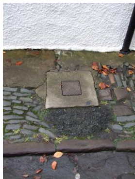
Poorly maintained historic surfaces, Backdykes 2009
