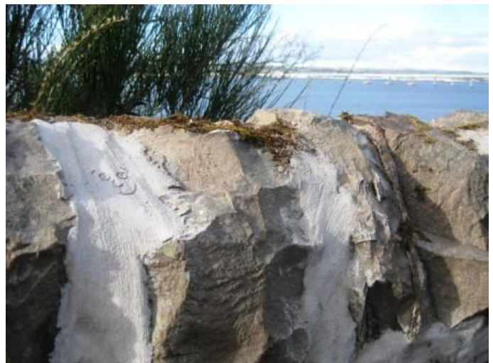
Re-pointed traditional rubble front boundary wall using modern cement mortar.
