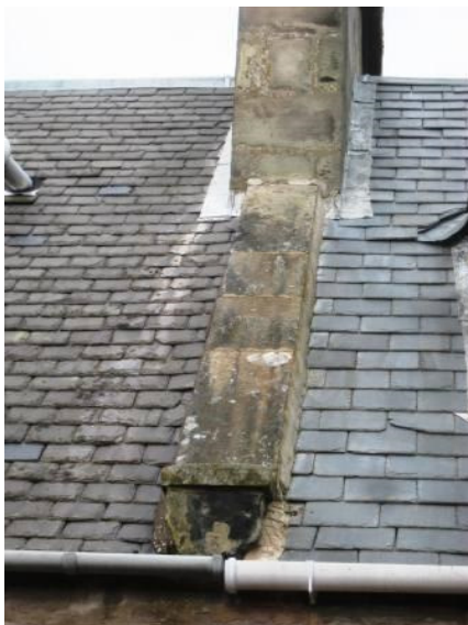
Original slate roof (left) replacement slate roof (right). Note also modern PVCu gutters.
