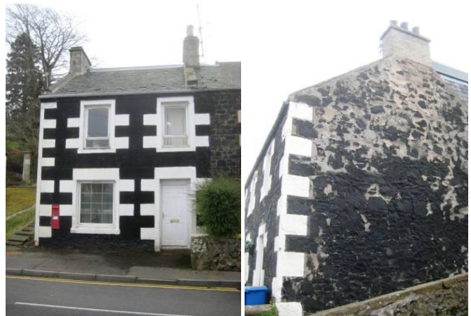
Traditional coal tar applied to exposed gable wall. Note inappropriate modern cement re-pointing.
