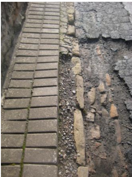
Modern pavement treatments and areas of damaged road surfaces revealing traditional materials and details
