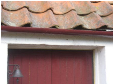
Door lintel, dated 1790 over-painted with modern film-forming masonry paint (Routine Row)
