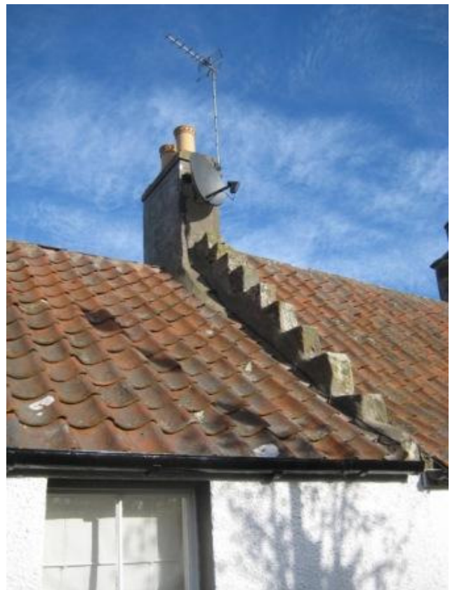
Satellite dish and aerial on listed building
