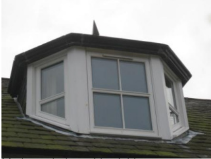
Modern window with trickle vents; imitation multiple pane glazing; sash and case; and glazing beading.
