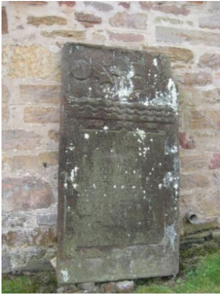
Cement rich mortars used for re-pointing the Category B listed Parish Church
