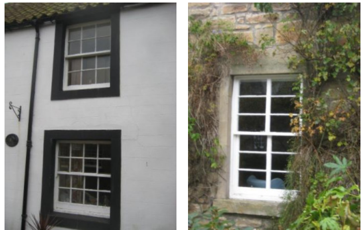
Examples of the wide variety of traditional window styles represented within the conservation area.
