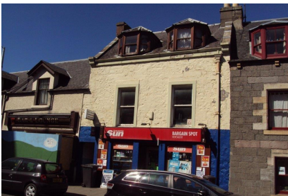
Peeling modern film-forming masonry paint.
