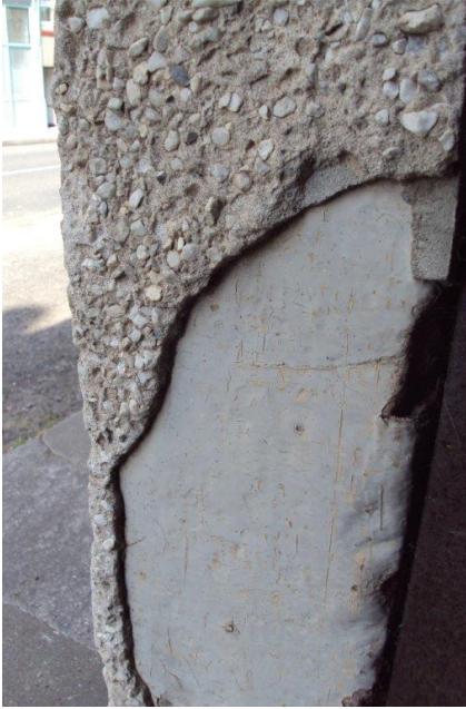
An example of typical failure of modern cement render applied to a traditional masonry wall.
