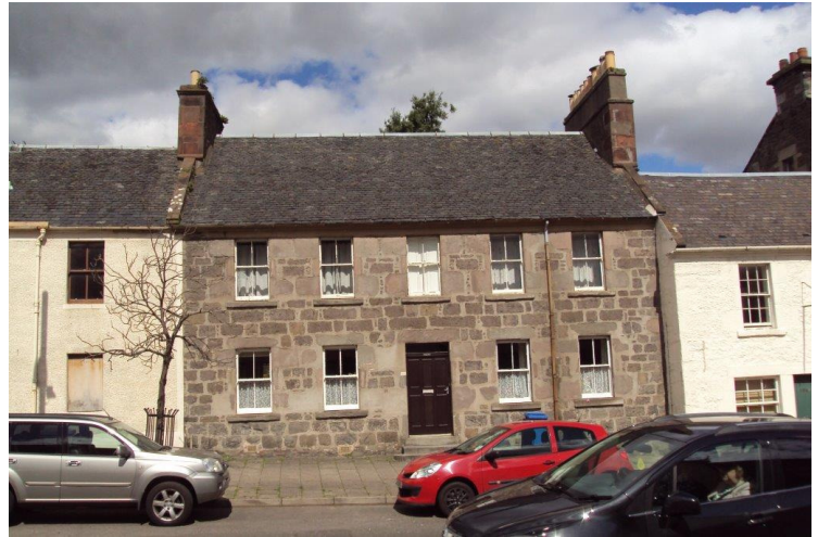
An example of the visual impact of inappropriate re-pointing.
