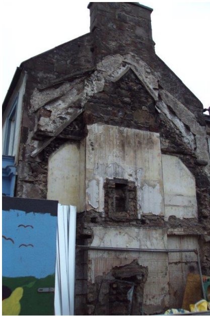
A recently exposed gable wall shows the changing roof pitch over time - from thatch, to raised eaves, to slate.
