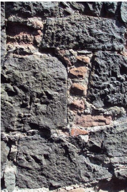
Some of the many traditional masonry styles found in the conservation area, using the local grey whin stone.
