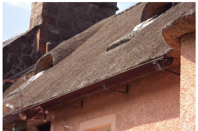
165-173 High Street. Restored by the National Trust for Scotland under the Little Houses Improvement Scheme.
