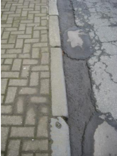
An example of poorly maintained road surface and inappropriate pattern and material used for the path
