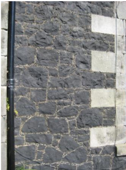
Example of typical traditional masonry - whinstone rubble with sandstone door and window margins. Note decorative 'cherry-cocking' in mortar joints.
