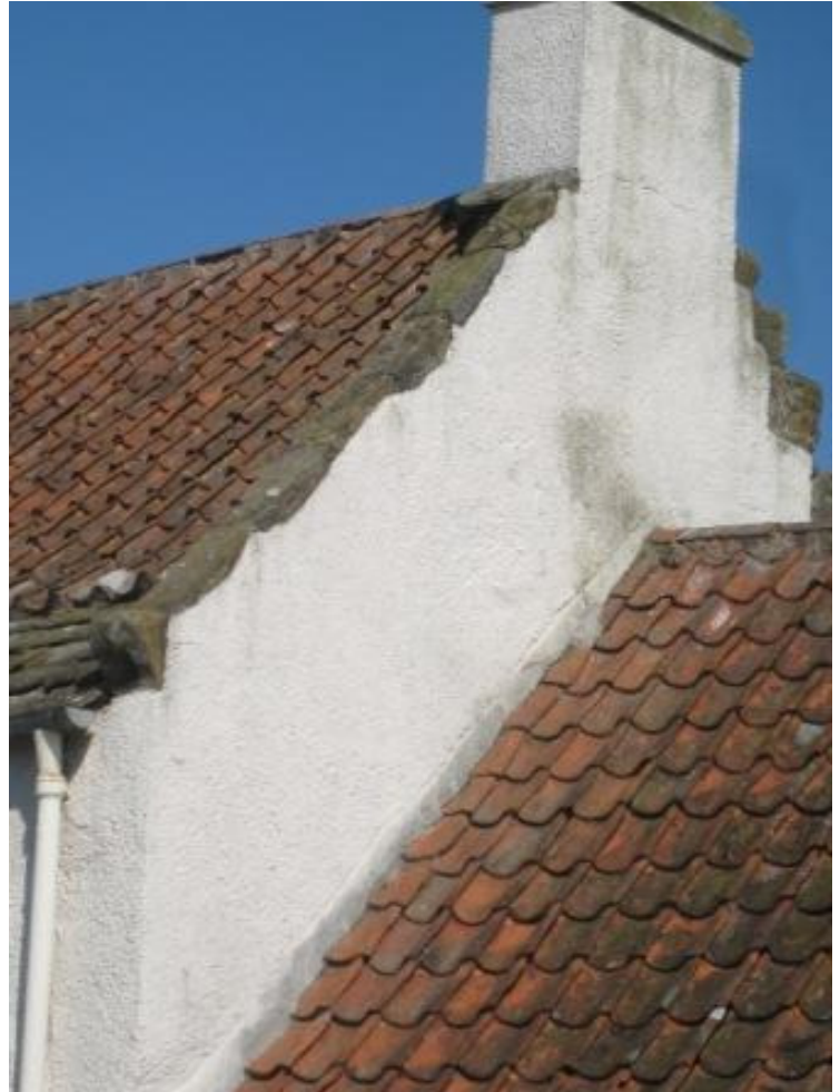
Example of typical East Neuk vernacular with pantile roof; slate easing course; carved skew-put; thackstone; stepped corbie gable, harled rubble walls.
