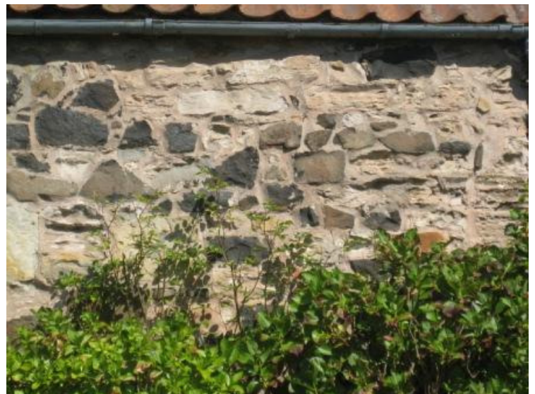
Use of modern cement rich mortars for re-pointing masonry
