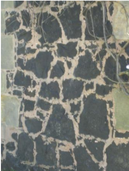
Decorative tightly pinned whin masonry joints ('cherry-cocking') obscured by unnecessary over-pointing
