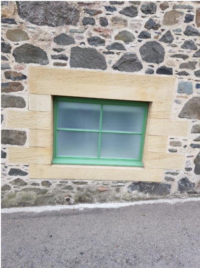
A modern (1954) window inserted into a gable wall. Recently, improved by renewing in more sympathetic traditional materials.
