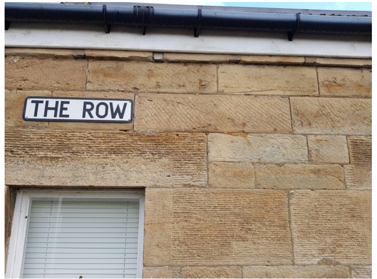
Broken random ashlar sandstone masonry.
