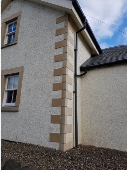
Inappropriate 'traditional' architectural detailing.
